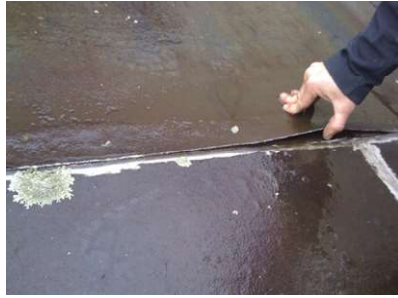
Example of a poor repair to a lap joint
